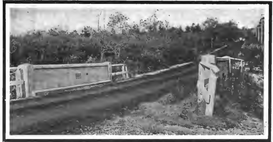
Culvert building has been revolutionized since the automobile stimulated the good roads movement
